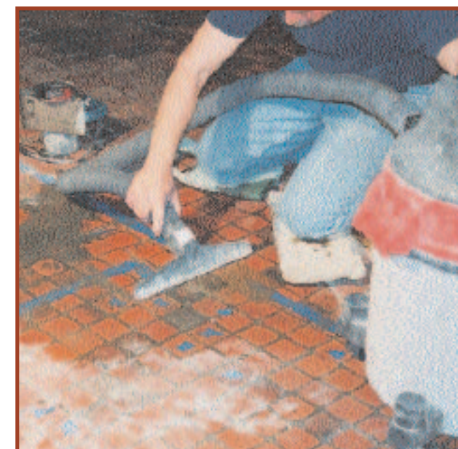
VACUUMING WATER FROM WET SAW USED IN CUTTING GROUT LINES AND REMOVAL OF WORN TILES
