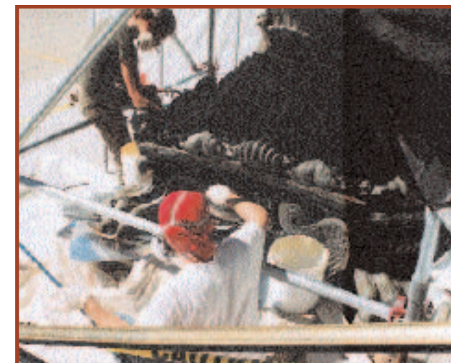
CONSERVATORS APPLY PATINA AND TINTED WAX TO BASE OF THE LIGHT STANDARDS LOCATED AT THE CAPITOL'S MAIN ENTRANCE
