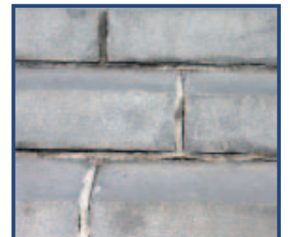
DETERIORATED MORTAR JOINTS
