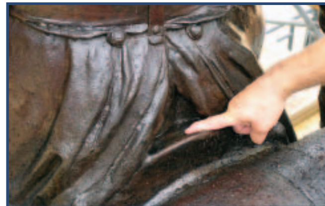
IDENTIFYING SOURCES OF WATER INFILTRATION
