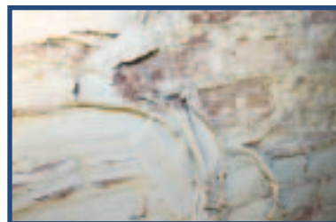
BASEMENT WALL MOISTURE DAMAGE
