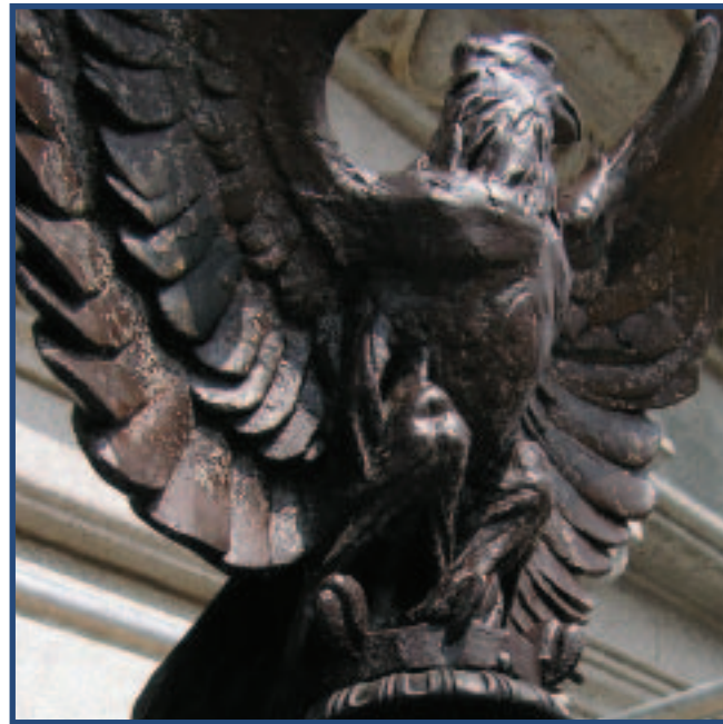
DETERIORATED CONDITION OF EAGLE ATOP LIGHT STANDARD
