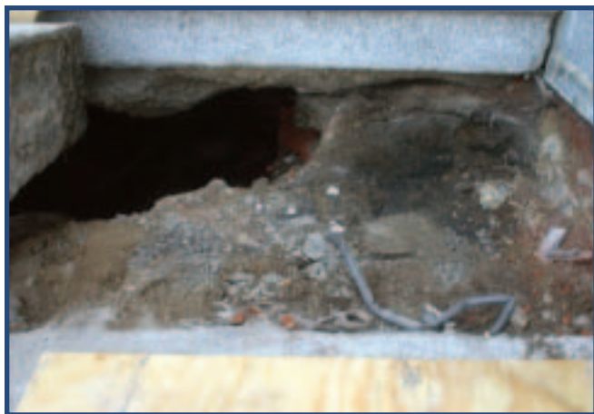
DETERIORATED FOUNDATION PIER SUPPORT
