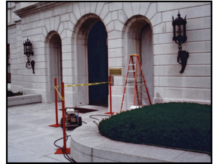
INITIAL SETUP FOR SAMPLE CLEANING APPLICATION AT THE MATTHEW J. RYAN BUILDING, EAST ELEVATION.
