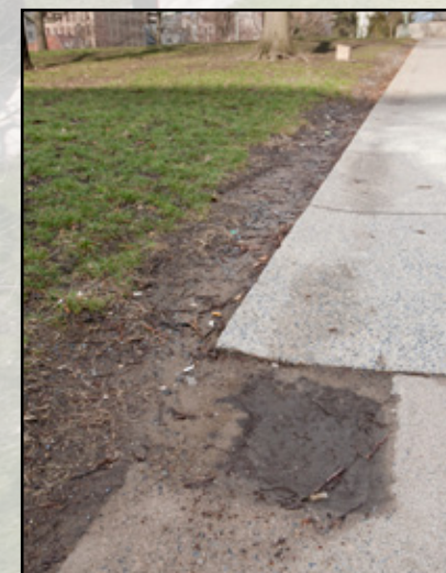
View of debris filled drainage pipe
