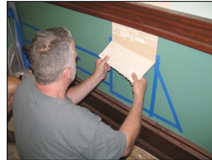
Section of the painted wall canvas being pulled back to install ductwork
