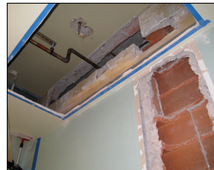
View of channeling in clay tile wall and suspended plaster ceiling for installation of new ductwork
