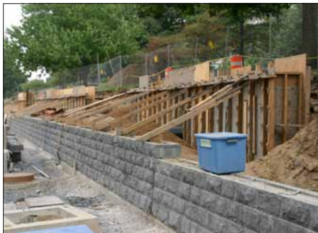
Western retaining wall with granite veneer and eastern retaining wall with poured concrete forms
