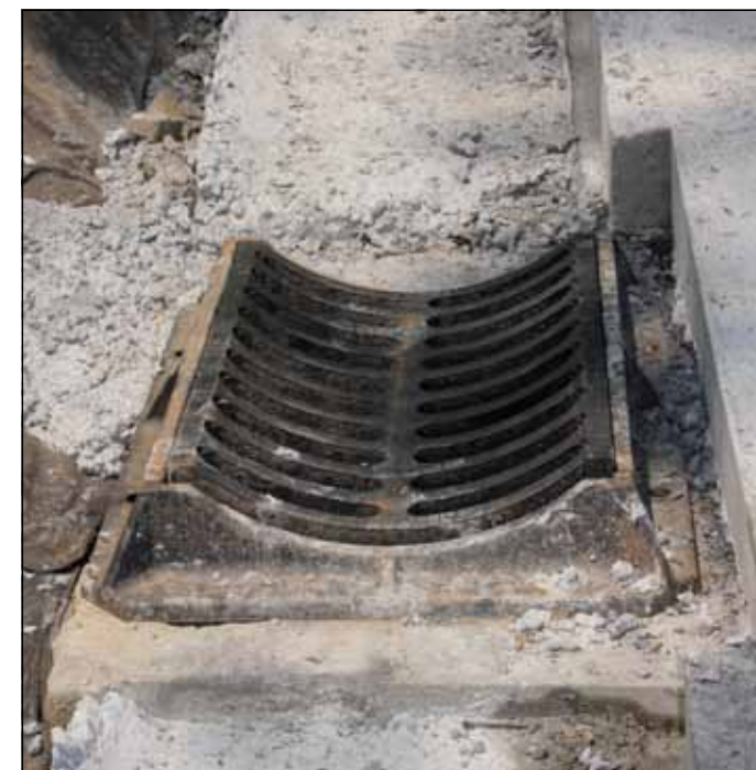
Concave inlet grate sitting on catch basin along interior park path prior to gutter installation
