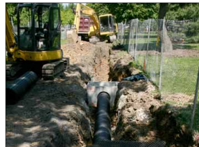
Catch basins connected by 15" pipe along interior park path
