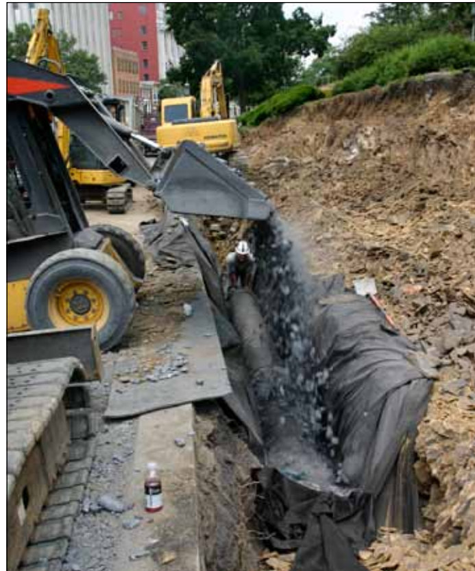
15" pipe on Third Street wrapped in geotextile fabric, back-filled with stone and wrapped in fabric again
