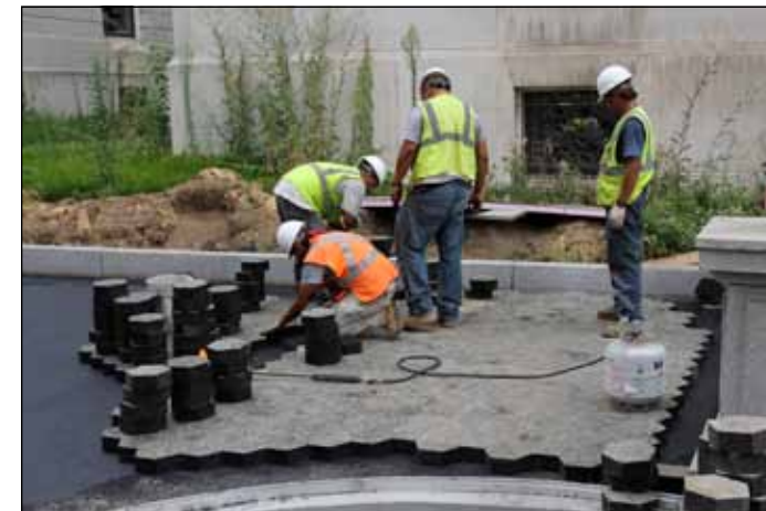
North interior park path with existing granite curb, asphaltic setting bed and partial hexagonal asphalt pavers
