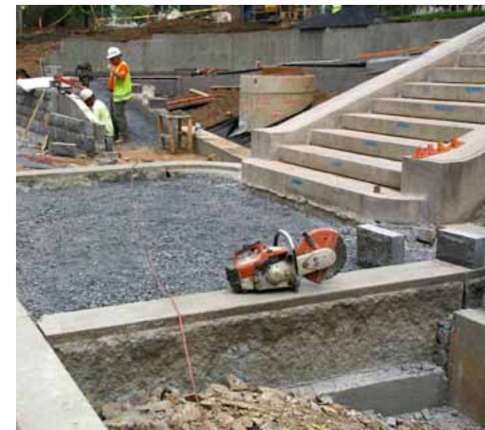
Partially reconstructed steps, footer, gravel bed for new sidewalk and granite curb Third Street
